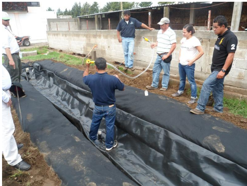
Figure 19 Biogas tubes are connected to the biodigester
