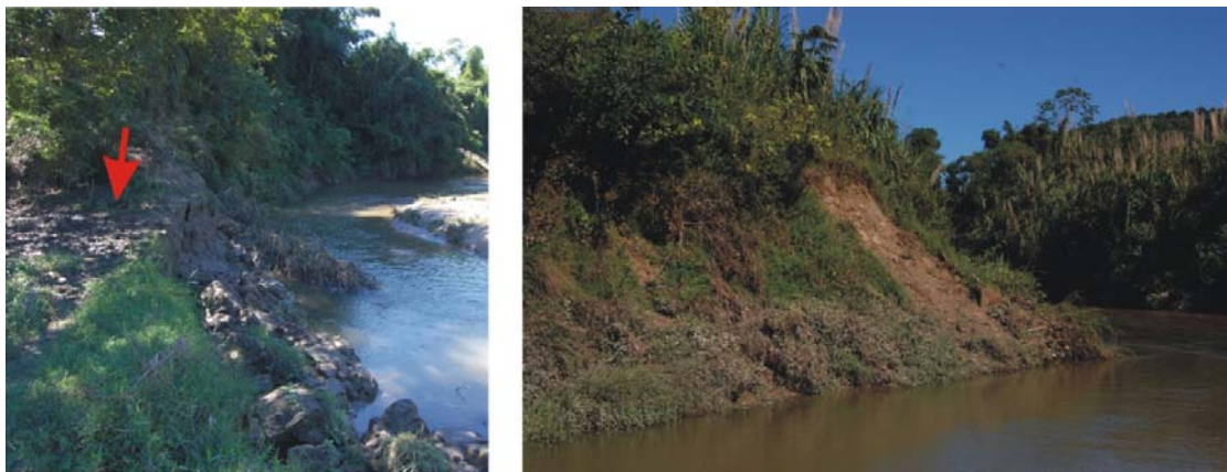
Figure 19: Examples of human-induced bank instability, both in Batatal river: cattle trampling (left, marked with an arrow) and channel modification (right).
