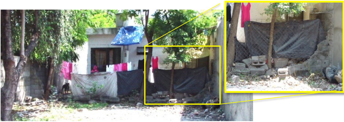
Image 23 2008 flash flood torrent was able to destroy a wall from a Magisterial suburb property (according to specialized informant) located between the two walkways from the suburb. Source: own
