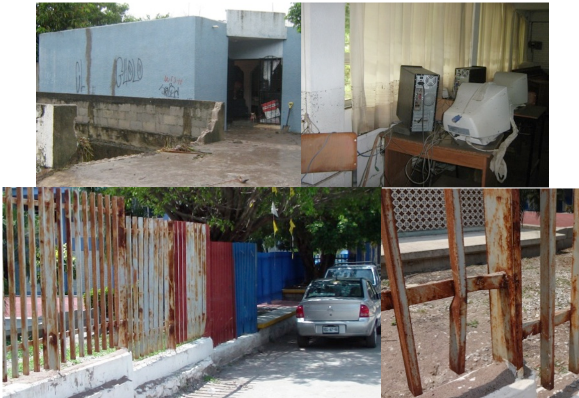
Image 40 Damages to public infrastructure (left); according to witnesses a floating cow destroyed this channel wall during the flood. The National Pedagogical University adjacent and immediately at the lower part of Magisterial suburb suffer great damage during the flood. Watermarks on the walls inside their library are visible and fence was blended by debris within the flash flood torrent. (photos from the bottom were taken at field survey 2014, own source)
