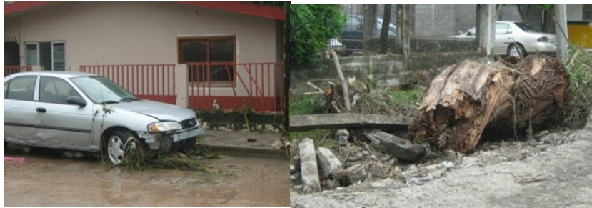
Image 33 Left: Damage caused to the fence and the car at the higher part of the city during the flood. Right: trees and light posts were completely broke and dragged by the torrent.
