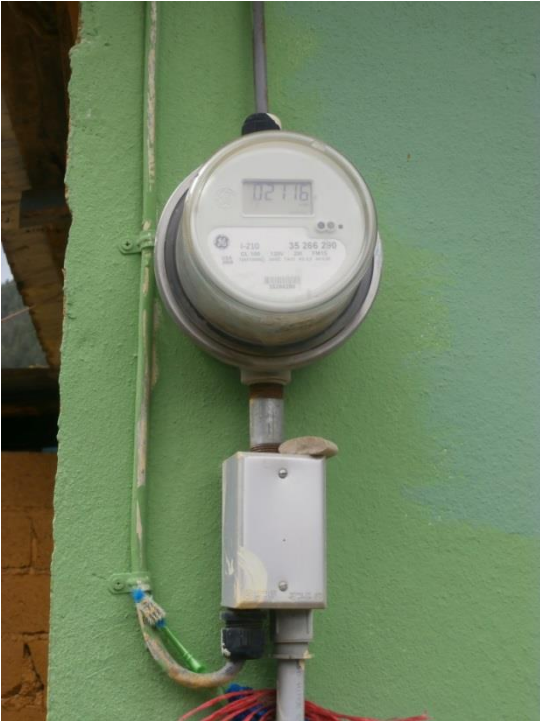
Photo 10. Consumption meters in each house Paso de la Perra
