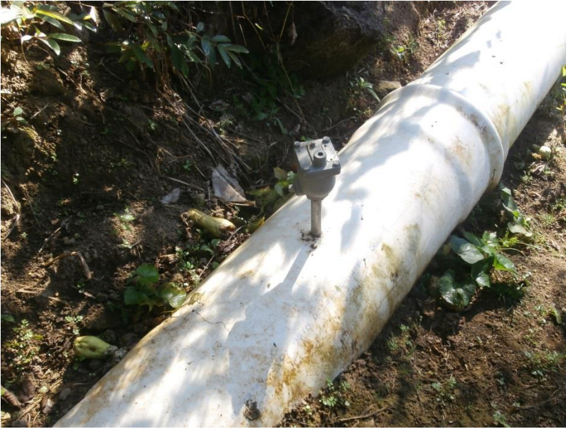
Photo 15. Valve in Pipeline Arroyo Frio
