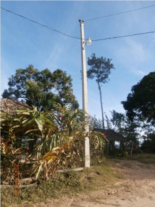
Photo 33. Grid lamppost in areas accessible by car Montazo-Valleicto
