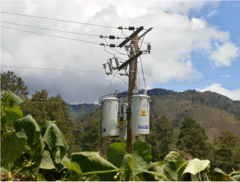
Photo 13. Transformers Arroyo Frio
