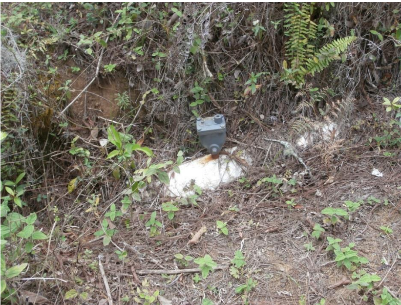
Photo 4. Valve in the pipeline Paso de la Perra
