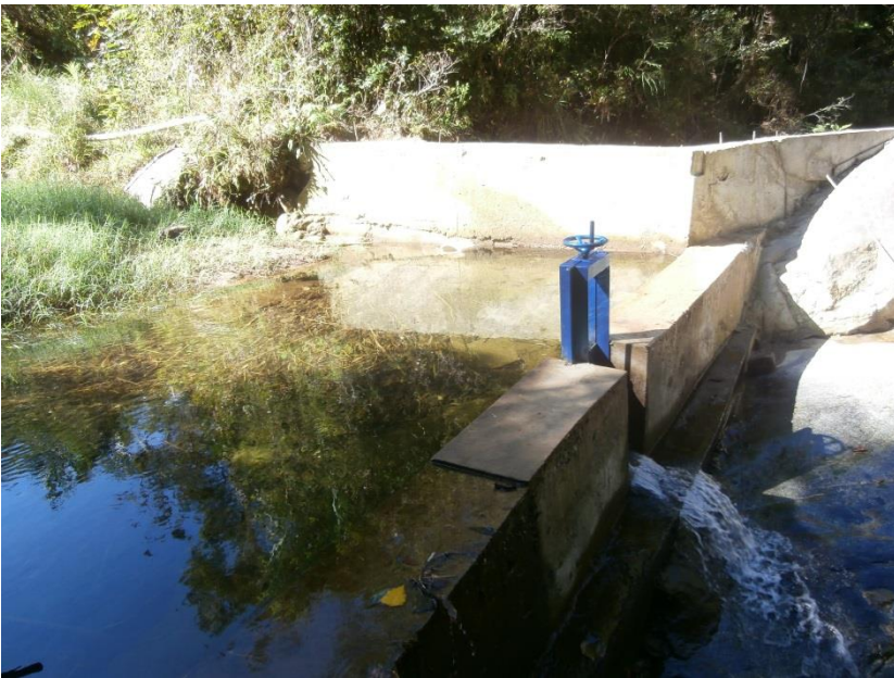
Photo 20. Water intake (ecological flow)
