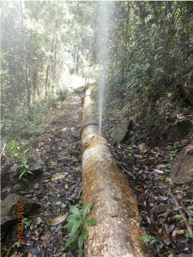
Photo 28. Not valves but holes Montazo-Vallecito
