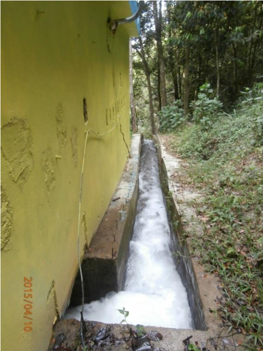
Photo 25. Water going out of the turbine Montazo-Vallecito
