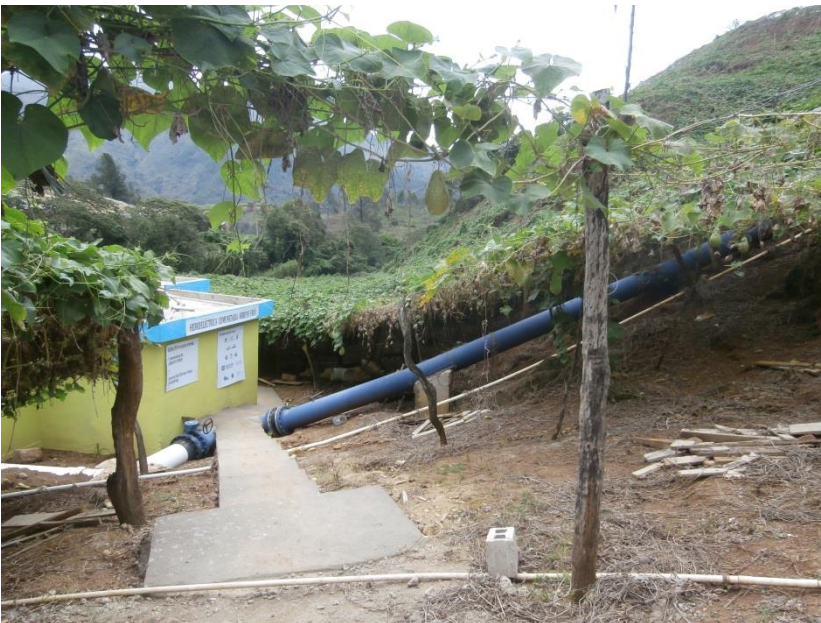
Photo 12 Power house Arroyo Frio
