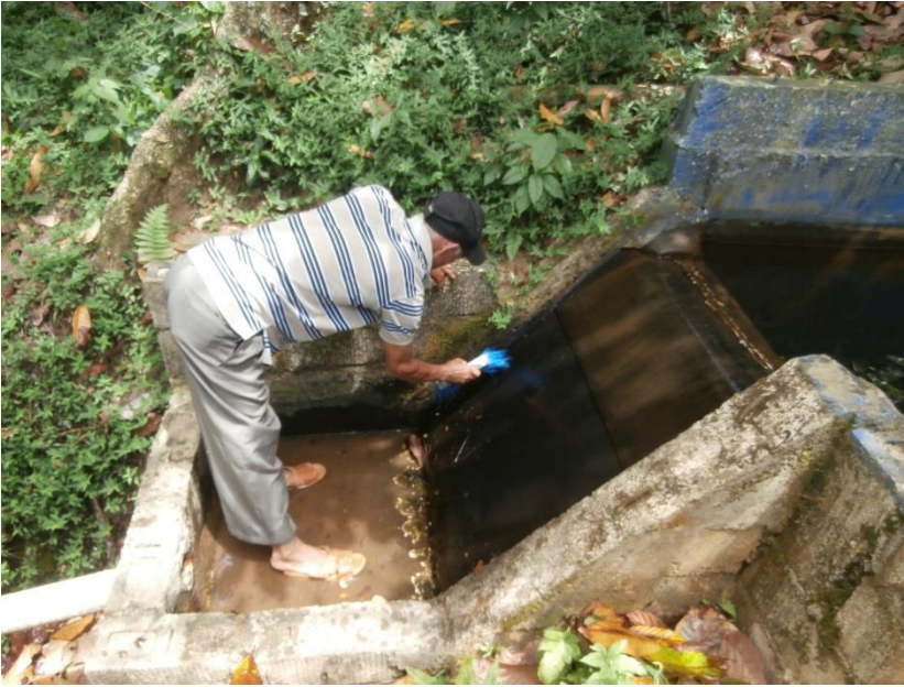
Photo 41. Grit removal Arroyo Majagua
