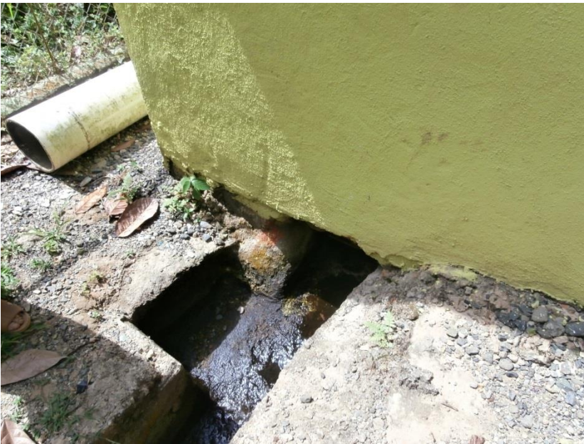
Photo 38. Water going out of the turbine Arroyo Majagua
