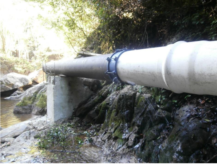
Photo 17. Joints iron-PVC pipeline Arroyo Frio
