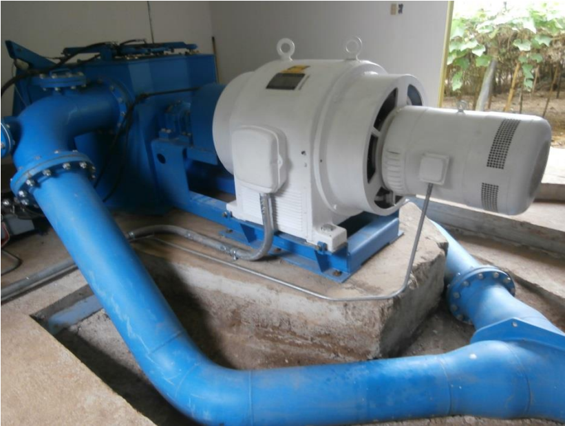
Photo 11. Equipment. Turgo-horizontal Arroyo Frio
