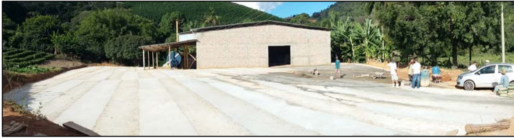
Figure 4 Concrete patio to dry coffee beans
